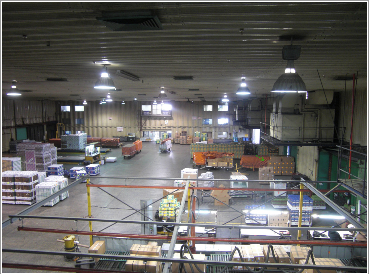
Airport perishables warehouse view. The majority of Israeli perishables exporters pack and dispatch their goods from this facility. Temperature in the facility is maintained at optimal levels by an industrial air-conditioning system designed specifically for handling fresh produce.
